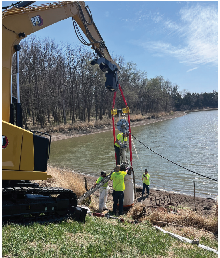
A crew slip lines a primary spillway on a dam in the Nemaha NRD. In 2024, the Nemaha NRD slip lined seven aging watershed structures.
