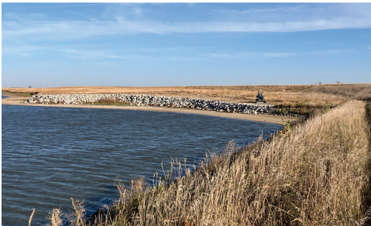
Little Blue NRD adds riprap to an earthen dam near Fairfield to prevent erosion.
