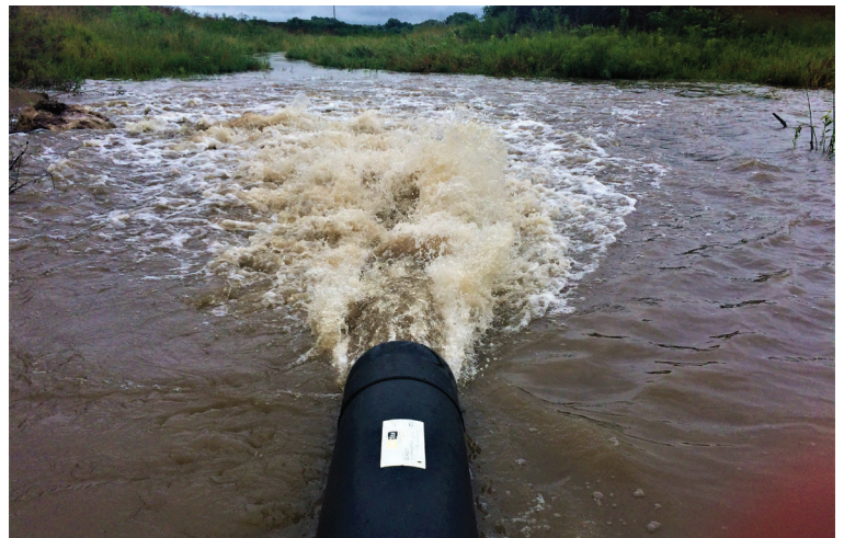
Water runs through Lower Big Blue NRD's Plum Creek Structure in Pawnee County, which was completed in 1979. The primary spillway of the 45-year old structure was recently slip lined.
