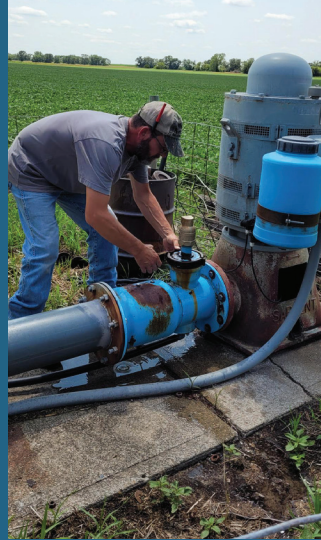
Middle Niobrara NRD Technician Travis Reagle opens a main line check valve during an inspection.
