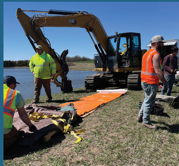
Crews prep to line the outlet of Lower Big Blue NRD's Cub Creek 10-C flood mitigation structure with a cast-in-place liner. The cost-effective repair involves inserting a flexible liner inside the existing pipe and hardening the liner. The liner forms a smooth surface inside the existing pipe, restoring it to near-new condition.
