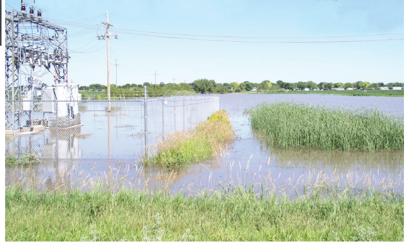
Heavy rains in July caused a substation to flood on the west side of Holdrege in Phelps County.
