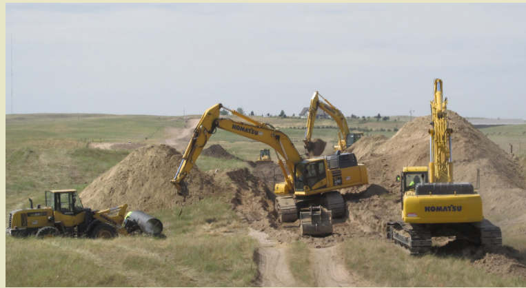
North Pipeline, NCORPE
