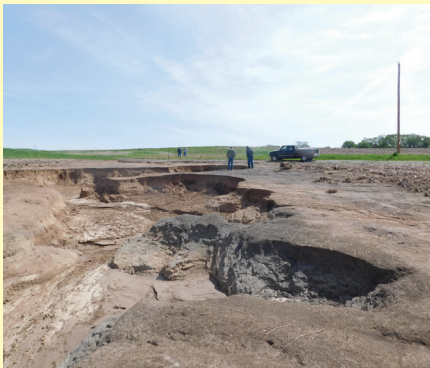
Flood Damage in Emergency Spillway in LBBNRD
