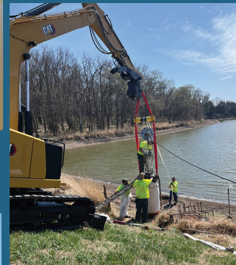
Below: A slip liner is installed on a Nemaha NRD flood reduction structure in May. Slip liners help prolong the life of aging dams. Over time, the corrugated metal pipe begins to rust and voids can begin to form under the principal spillway causing undercutting and potentially failure of the dam to function properly.
