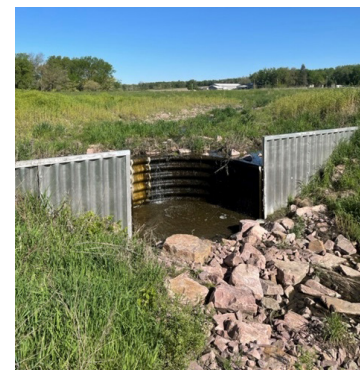
Lower Platte North NRD Landowner Tom Sprunk, located in the Shell Creek Watershed, worked with the LPNNRD and NRCS, with funding from NDEE, to place a toewall structure in a wetland pasture. The structure will help with the flow of excess water and improve streambank stabilization.
