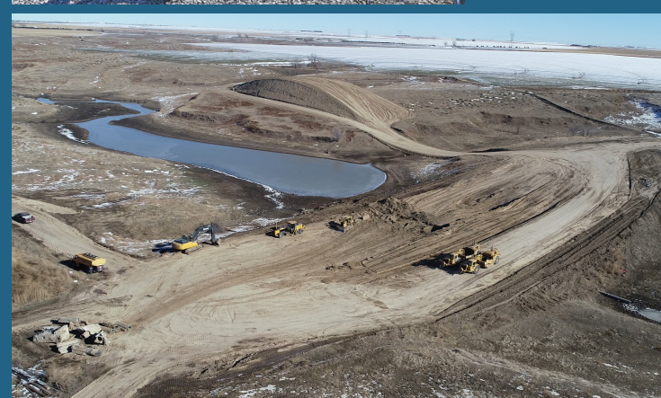
Middle Republican NRD's flood control dam (P2) near Culbertson is being rebuilt after it was damaged.
