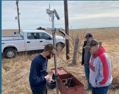
Lower Big Blue NRD Data Specialist Nick Schroeder, left, installs telemetry in dedicated monitoring well #18 near Diller with Ken Quandt of McCrometer, right.
