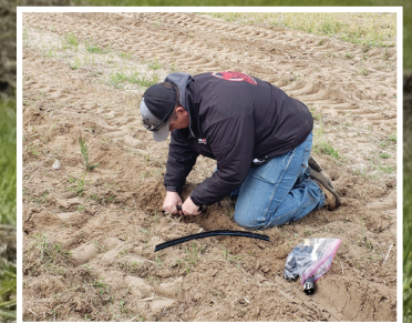
Tri-Basin NRD Land Resources Manager Nate Munter installs fittings in a drip system for a 2021 tree planting.
