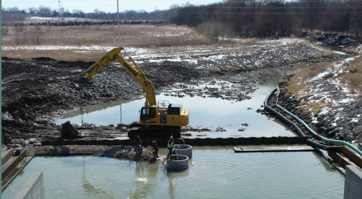
Lower Platte North NRD continues work to repair the Lake Wanhoo stilling basin. This damage was sustained during the 2019 floods.
