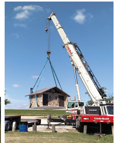
Upper Big Blue NRD recently installed upgraded bathroom facilities at Smith Creek (Utica) and Oxbow Trail (Ulysses) recreation areas.
