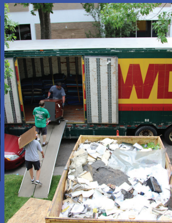
SERVPRO moves out NARD office furniture to determine if it can be cleaned and salvaged.
