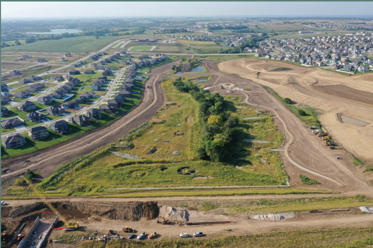
Papio-Missouri River NRD's new flood mitigation reservoir, Big Elk Lake, takes shape in Papillion. The lake will be fed by West Papio Creek.
