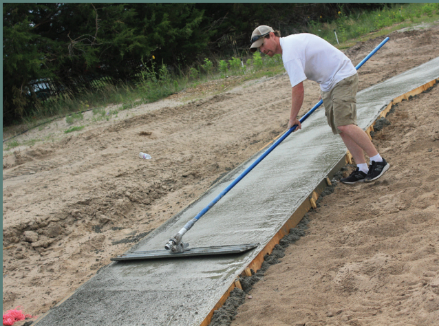
Above: Upper Loup NRD Resources Technician Shane Young smooths cement for a walking path at the new Arboretum in Theadford near the District office.
