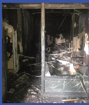
The first floor entryway to Inland-Insurance building shows extensive burn damage.
